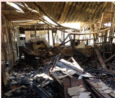
The old store after fire gutted the building
