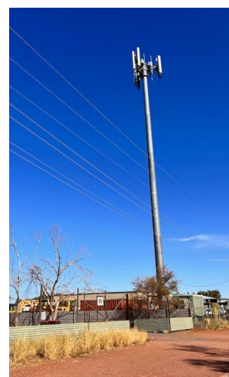
Figure 10: Mobile phone tower on Maloney Street, Tennant Creek.
