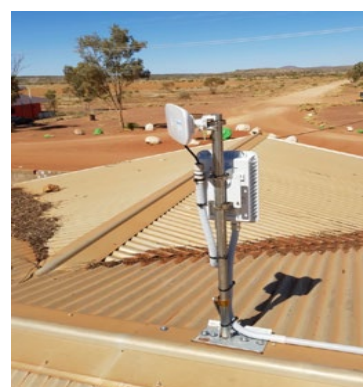
Figure 8: Wi-Fi Outdoor access point (Photo courtesy Easyweb Digital)
