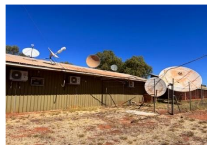
Figure 10. The huge old Tanami Network satellite dish is one of array of satellite dishes behind the PAW Media studios in Yuendumu
