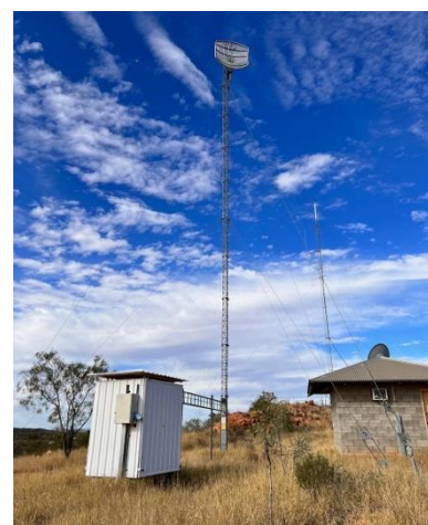
Figure 6: The 4G small cell tower has been installed in Yuelamu, awaiting backhaul connection.
