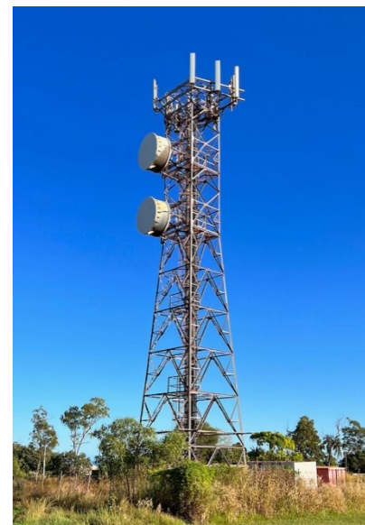
Figure 5: Mobile base station with microwave links to mainland
