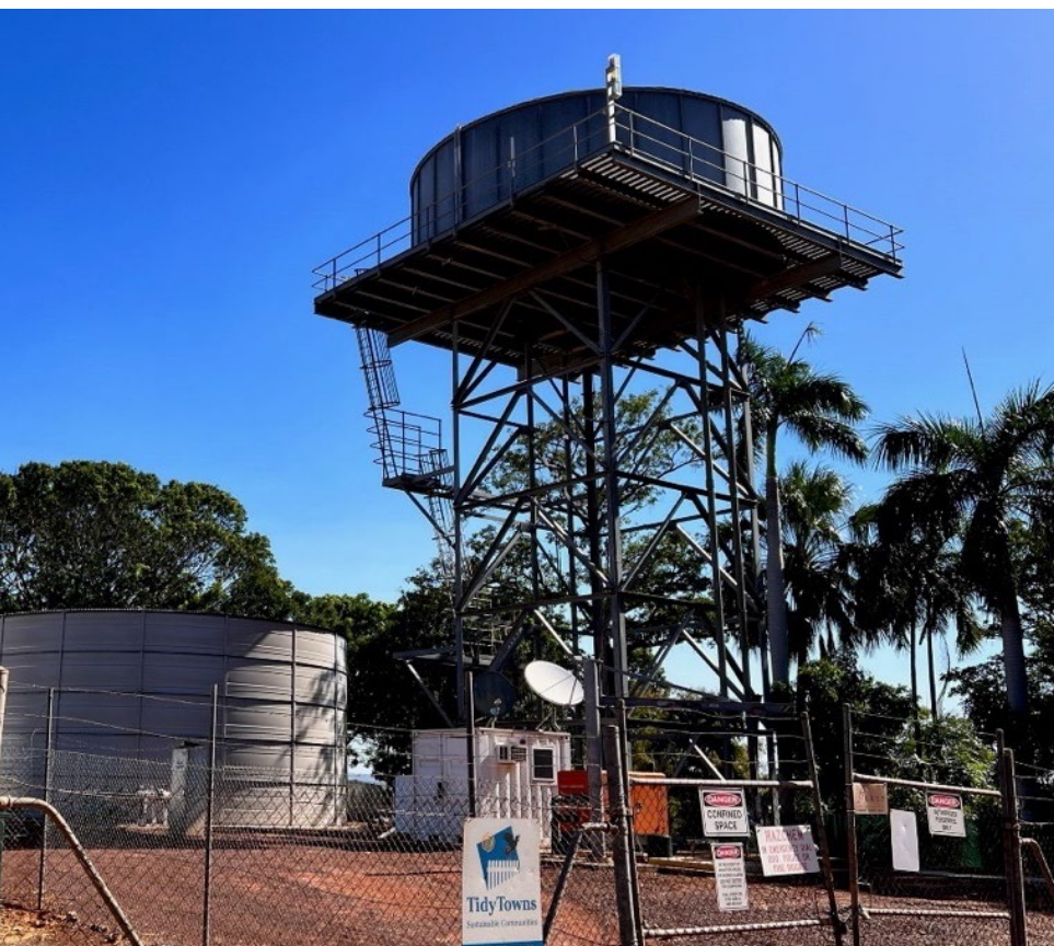
Figure 5: Telemetry is being used to monitor water tank levels, pumps, generators and other municipal services in many communities, however this relies on 4G or satellite backhaul services working effectively.
