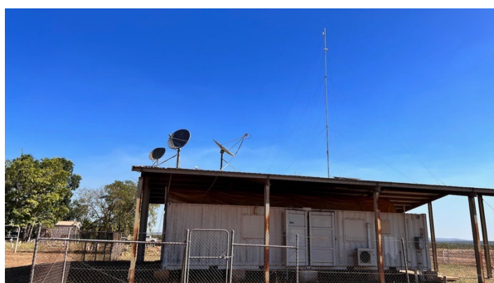
Figure 8: Access points are located on community buildings to enable line of sight connection to all houses.
