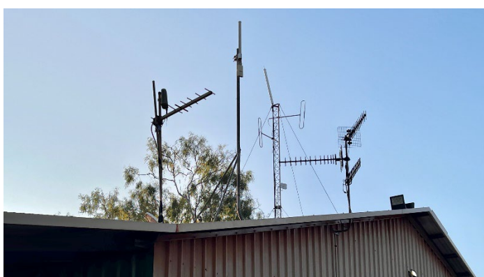
Figure 7: The DAC office roof is festooned with an array of communications transmission and repeater equipment.
