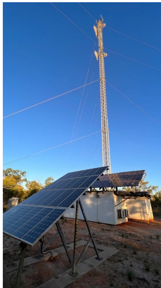
Figure 10: The 3G/4G macro-cell mobile tower is located near Cape Leveque Rd, 3.6km south of Djarindjin, however coverage is patchy within Djarindjin and Lombadina.
