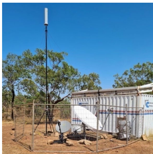
Figure 10: Temporary 4G satellite small cell mobile tower at Fossil Head
