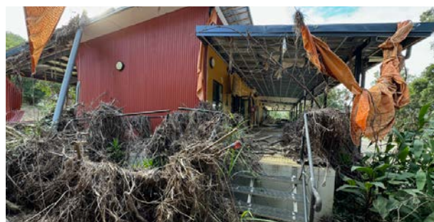
Damaged Bana Yirriji Arts Centre in Wujal Wujal; image taken five months after flood
