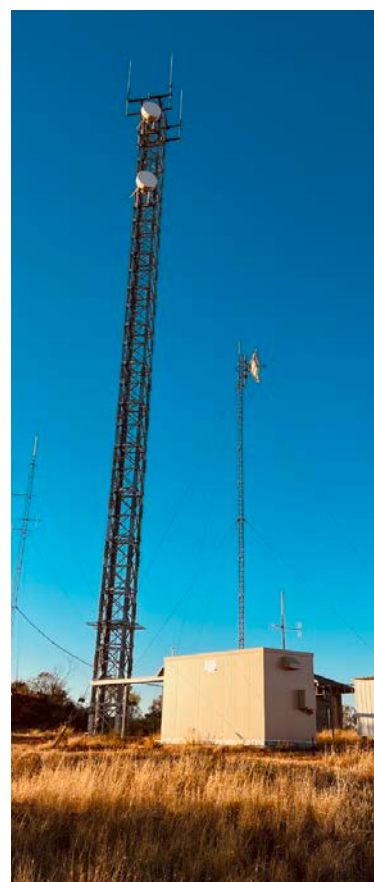
Newly activated 4G tower in Yuelamu
