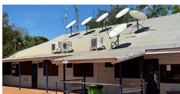
Sky Muster dishes on top of Kalumburu community office; four of which provide the backhaul for the mesh network
