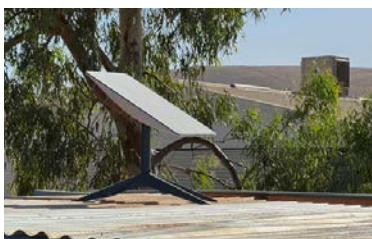
Starlink dish on top of house in Warakurna
