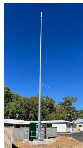
Figure 6: 4G small cell tower near hospital
