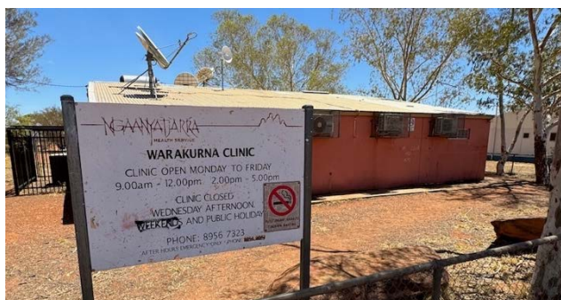
Figure 24: Warakurna clinic has old satellite dishes on the roof, since replaced by fibre connectivity
