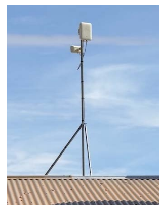
Figure 36: Access points are distributed on rooftops
