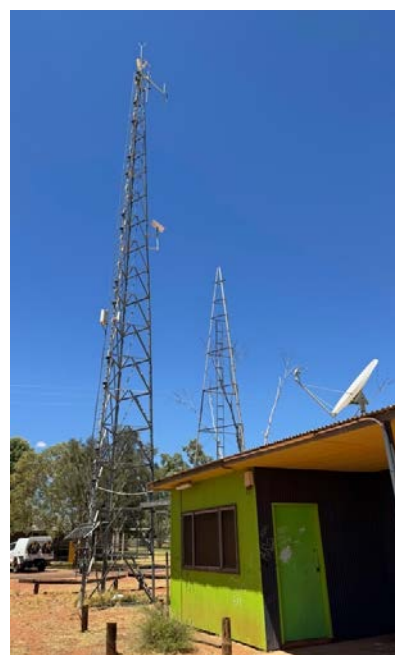
Figure 28: RIBS broadcast tower at Warakurna media centre could be used for digital TV broadcast
